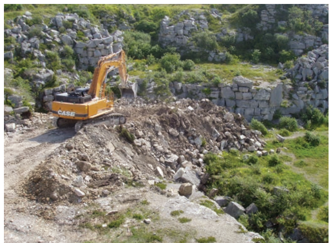
Figure 6. Construction of a new haul road for Jordans Mine which involved the importation of several hundred tonnes of spoil from the nearby Fancy Beach Quarry.
