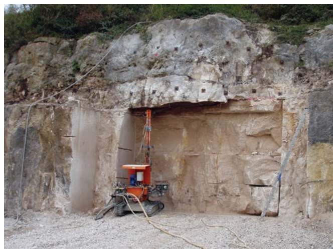
Figure 11. The wedge-shaped first advance of Jordans Mine and Marini bolting rig being used to install rock bolts into the newly exposed area of roof.
