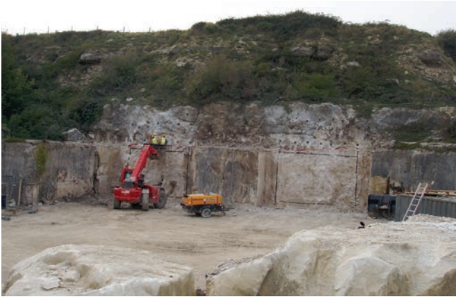
Figure 7. The installation of 30 horizontal rib-bolts designed to stabilize the immediate roof beam over the newly cut portal rebates was undertaken from a man-cage attached to a telescopic-handler.
