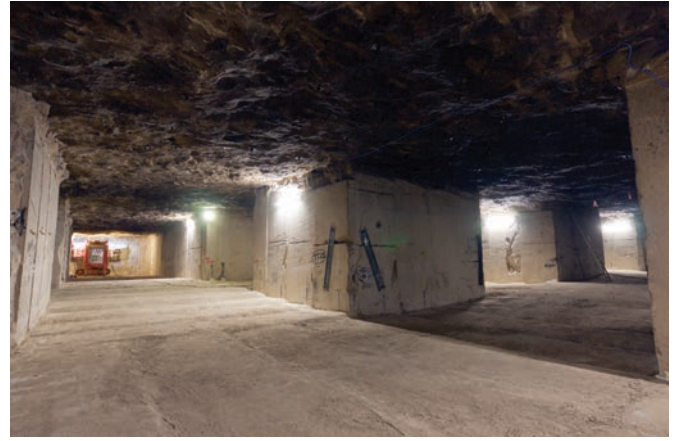
Figure 14. A jointed pillar which has been stabilised using rib bolts and cell straps.
