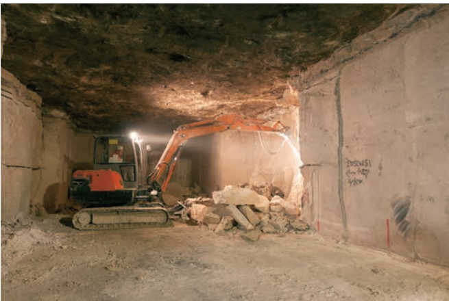
Figure 15. Trimming irregularities from a mine face using a backhoe fitted with a hydraulic breaker.
