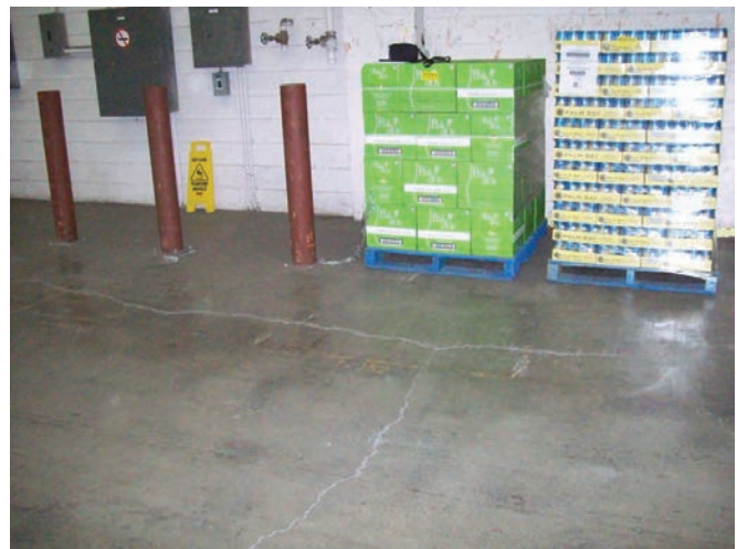
Figure 7. Intersecting floor cracks indicative of upward heave of the floor slab in a warehouse building in the City of Ottawa.
