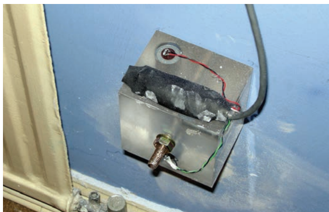
Figure 8. Tri-axial array bolted onto ground floor wall.
