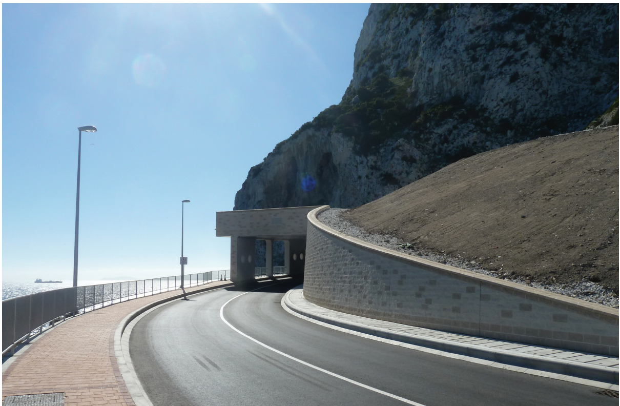
Figure 11. The completed rock fall canopy, counterfort retaining wall, rock fall catch ditch and approach road.
