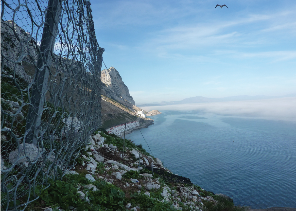
Figure 8. Completed rockfall catch fences. View looking north to Sandy Bay, Catalan Bay and the North Face.
